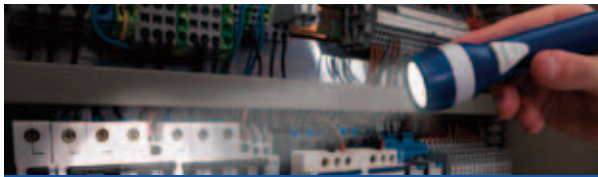
Erroneous circuit-breaker activation
